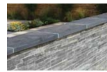
8: Parapet: Slate/Granite coping stone surround to edge of parapet. Colour to match local vernacular.
