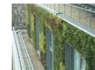
7: Living Wall. Plants to be Evergreen and suitable for Wet conditions. Plant species to be determined
