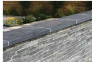
Slate/Granite coping stone surround to top of stone wall. Colour to match local vernacular.
