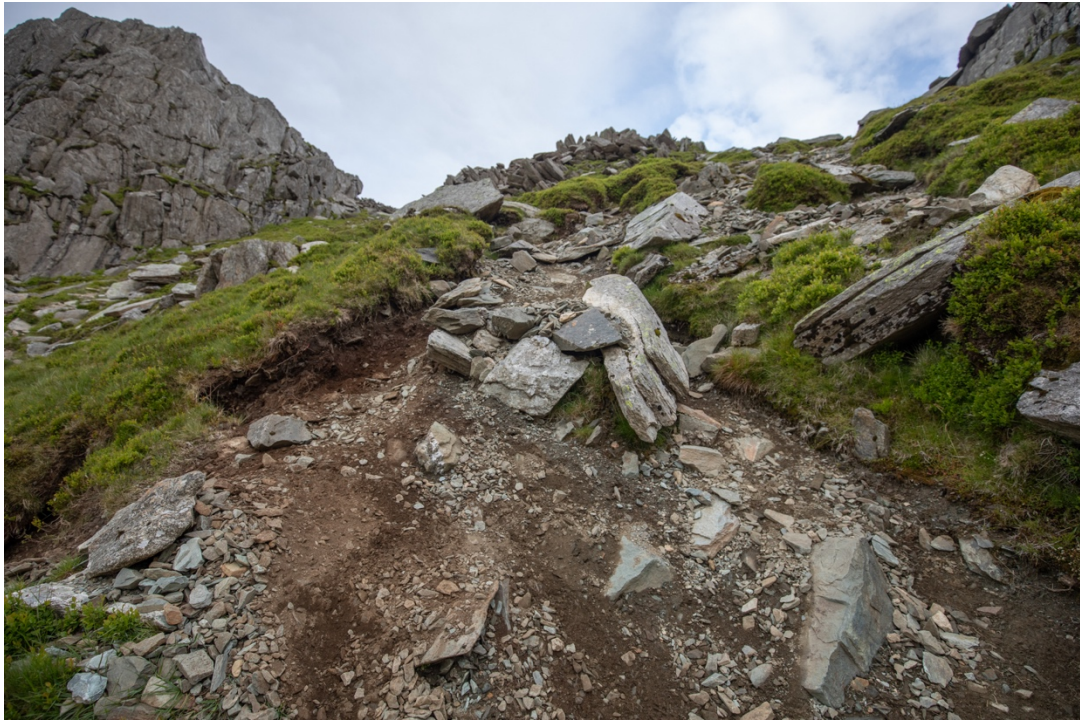
Above: footpath erosion near Tryfan along the 'heather terrace' at SH 66381 59182.
