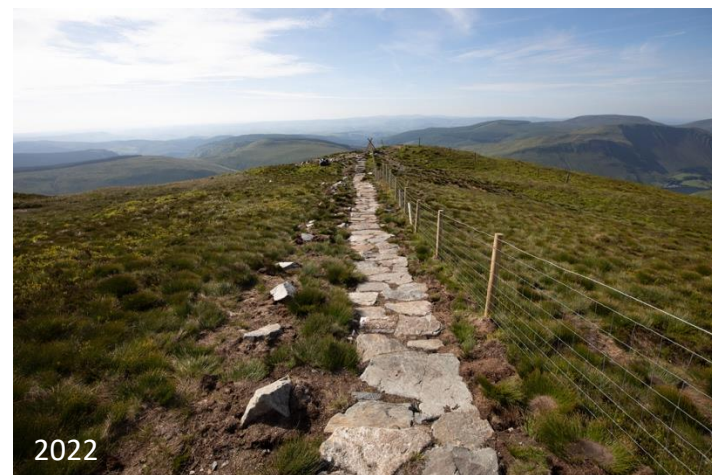
Image location: on descent from Mynydd Moel towards Nant y Gader ( P13 ); note new laying of hard core on this section pathway.
