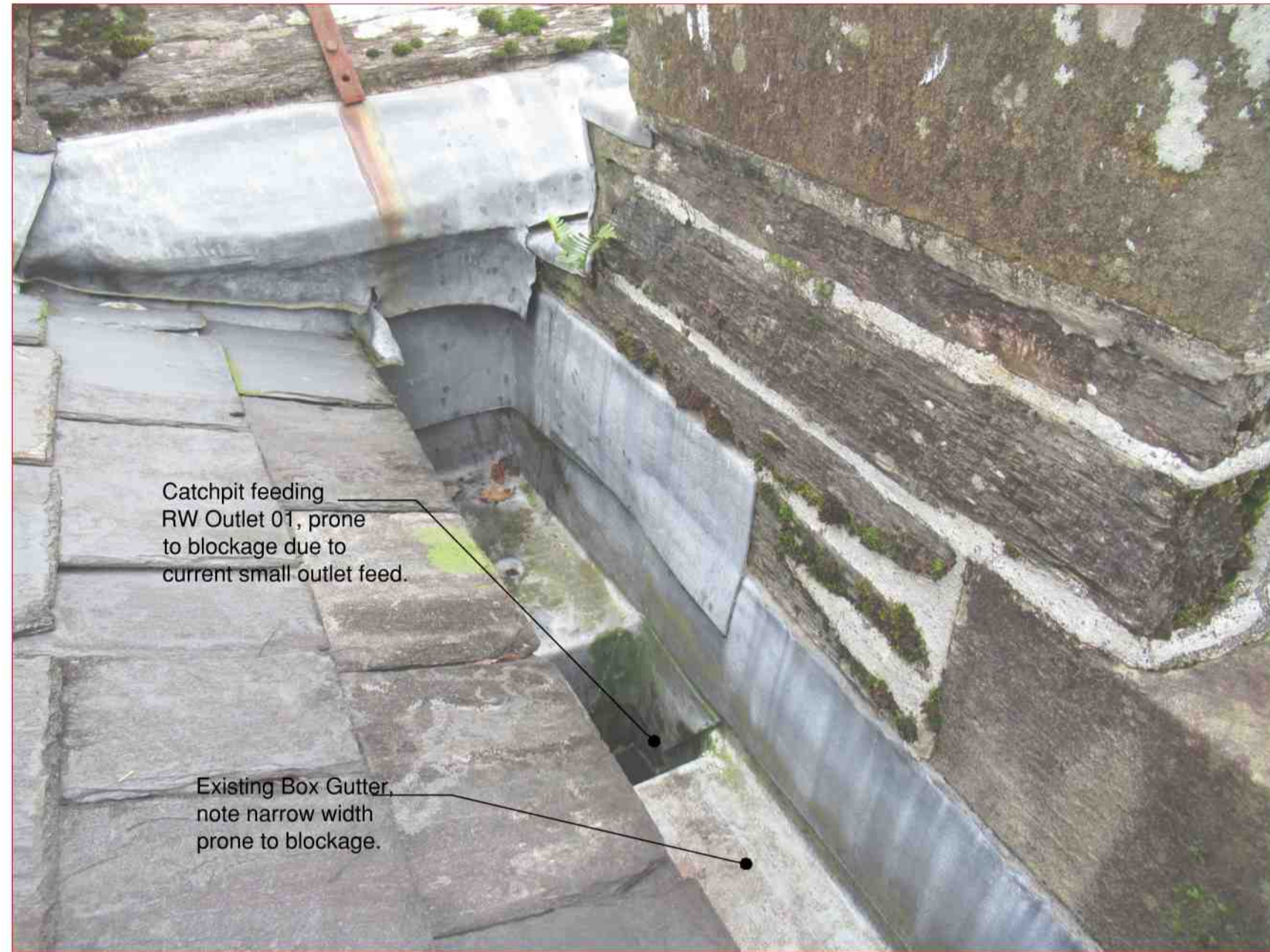
Photo of Existing Catch Pit Serving RW Outlet 01 from Roof Slope R3 (Photo 5761)
