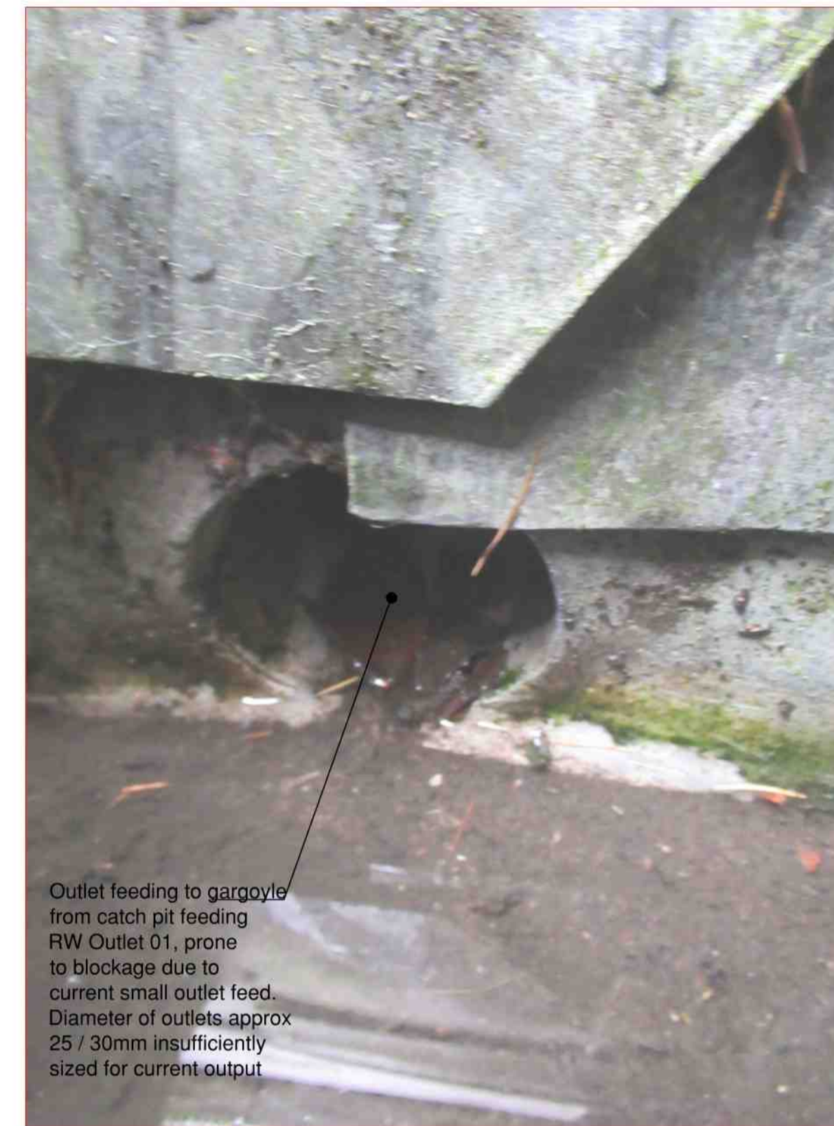
Photo of Existing outlet within catchpit Serving RW Outlet 01 from Roof Slope R3 (Photo 5766)
