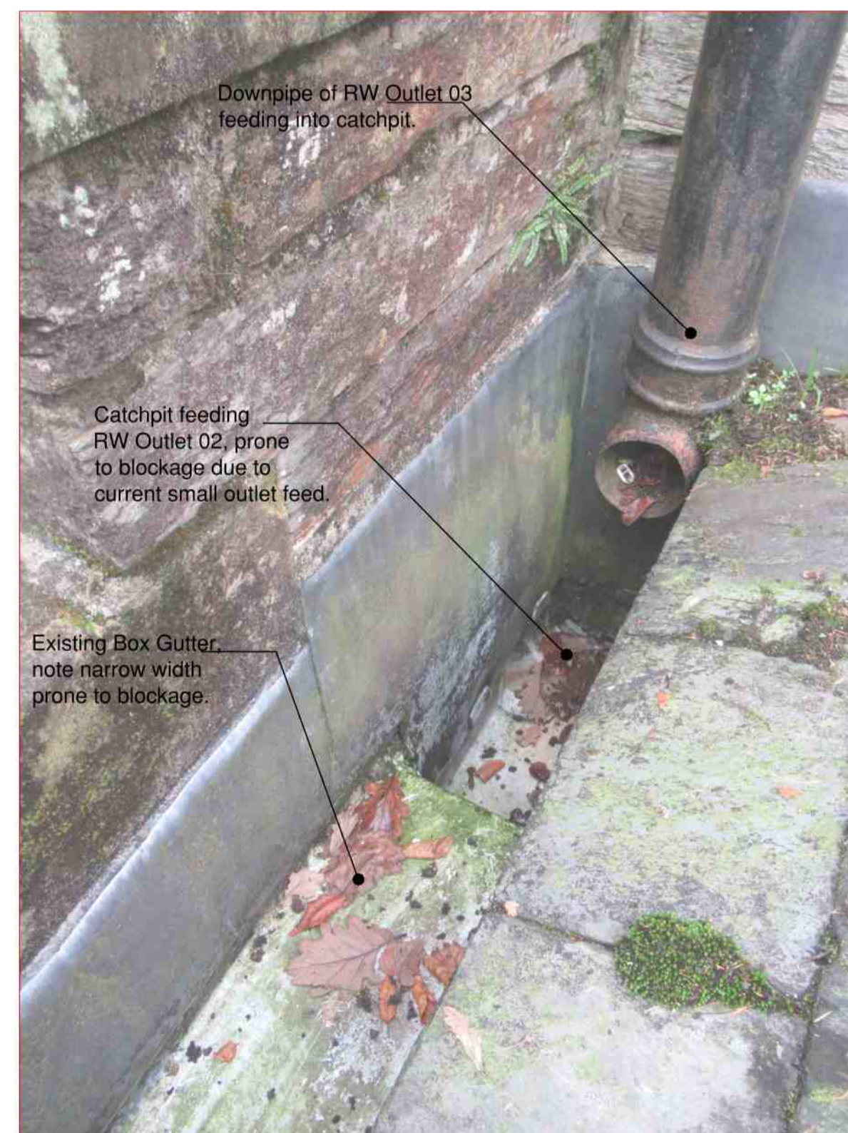
Photo of Existing of catchpit Serving RW Outlet 02 from Roof Slope R6 (Photo 5796)
