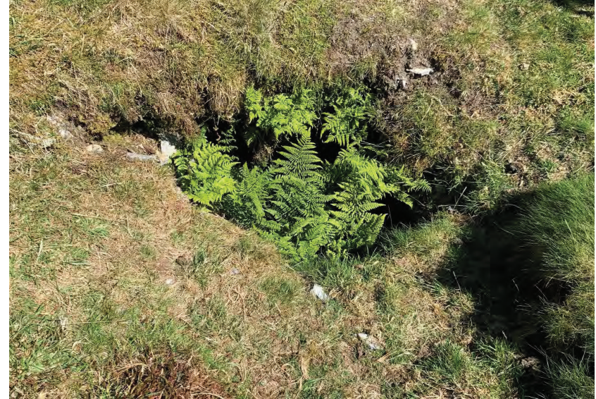
35. The opening in the ground that may be the result of settlement of backfill within a former mine shaft
